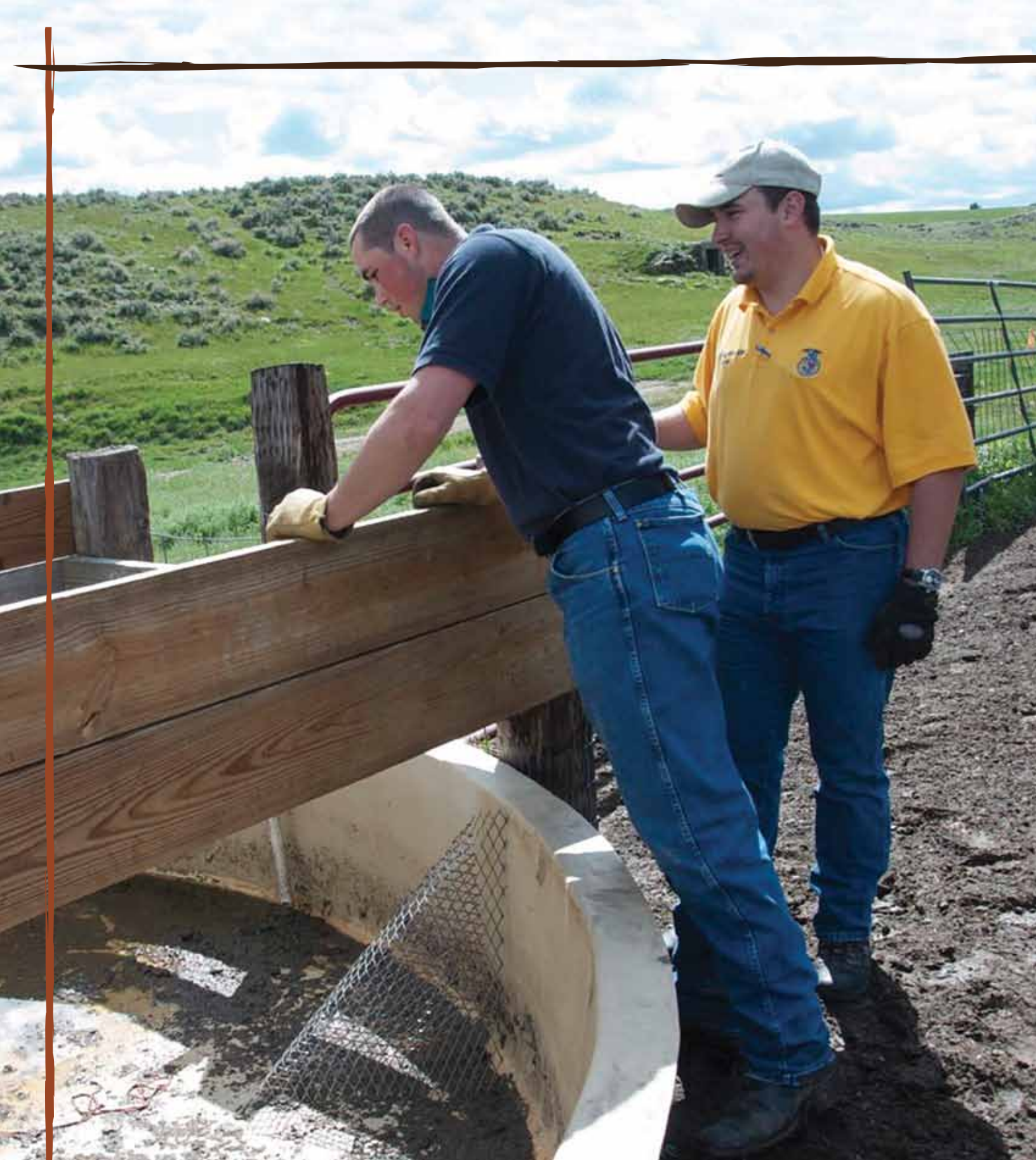
Volunteers retrofit livestock water tanks to add escape ramps for sage grouse and other wildlife.
